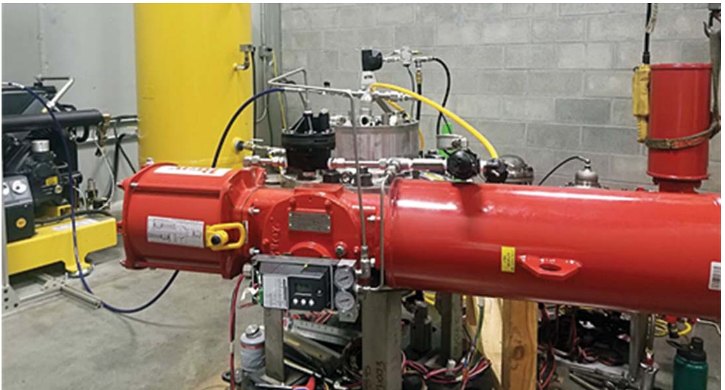
Photo of Validation Testing – Live Video and Live Data were streamed continuously for real-time monitoring of performance of assembly, sub-assembly and components.
