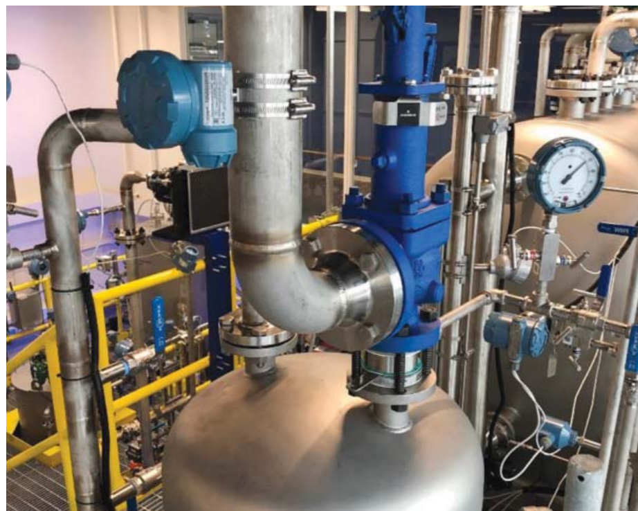
Figure 4: An acoustic transmitter (blue device in the upper left of the photo), can be mounted on the discharge pipe of a PRV, allowing it to detect the vibrations caused by any release. These devices send data via WirelessHART
