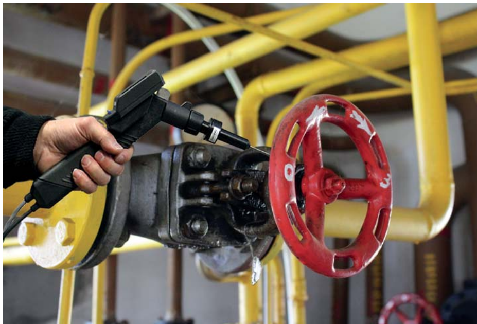
Fugitive emissions testing.
