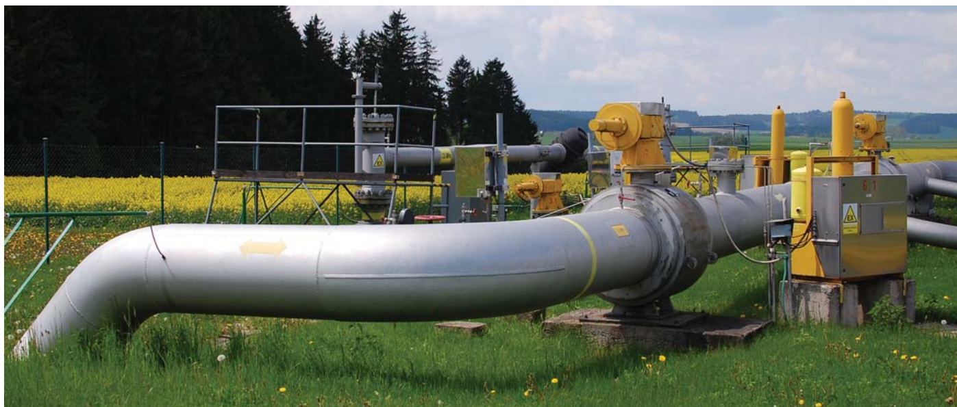
Pipeline safety studies show that blends containing up to 20 percent of hydrogen can be safely injected directly into the gas grid.
