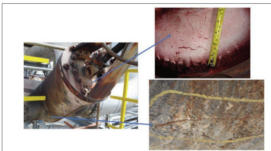
Figure 2: Cracks observed on the valve 12 .
