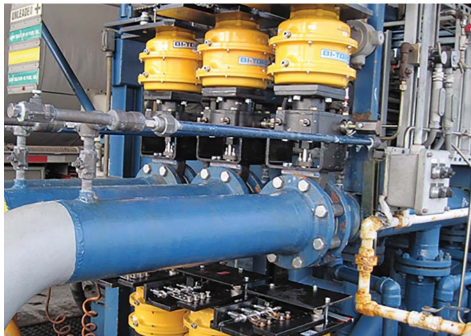
Bulk loading stations at a refinery.
