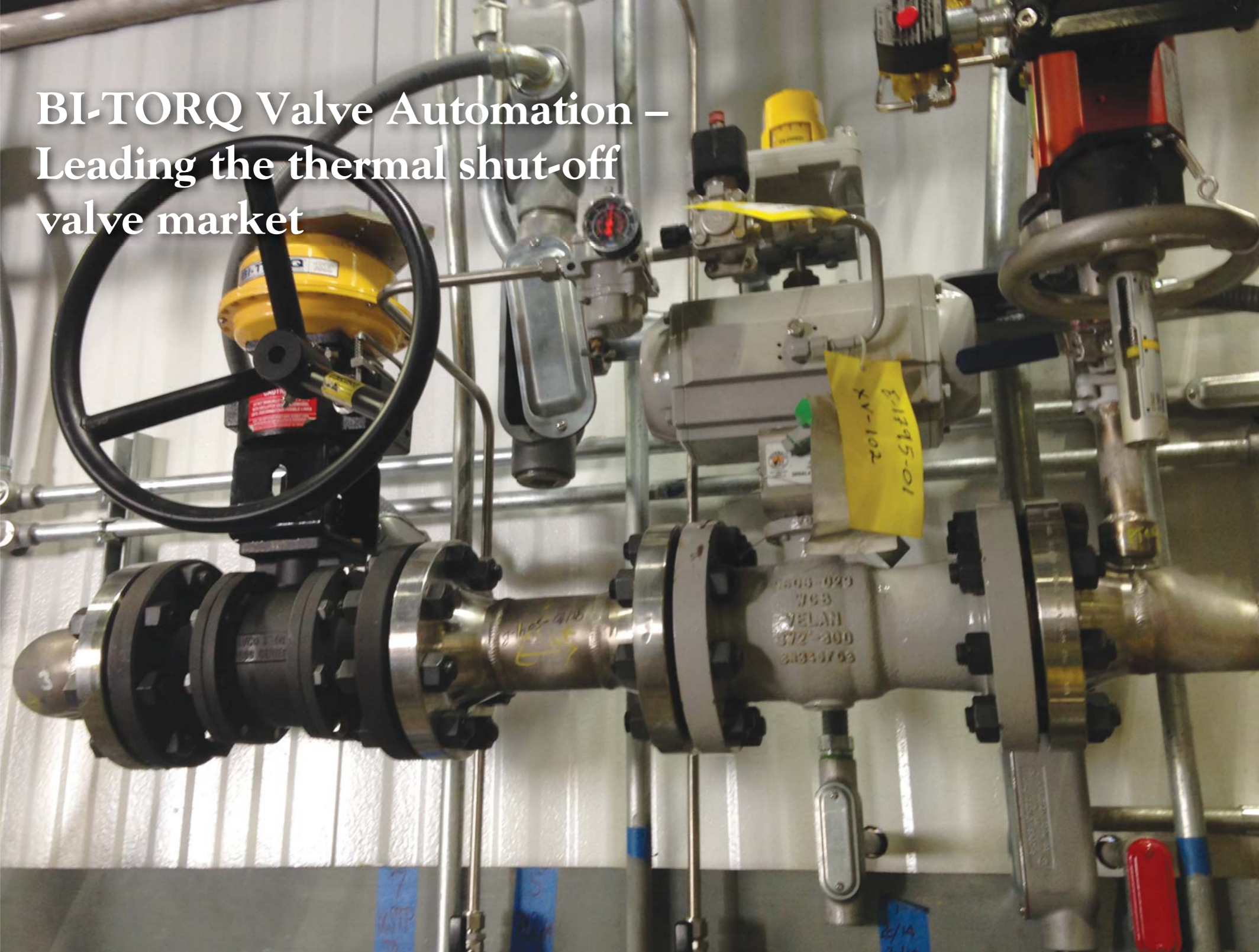
High pressure natural gas turbine installation.
