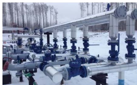
CIRCOR Energy | KF Valves ball and check valves installed and operating at an oil & gas facility in Canada.
