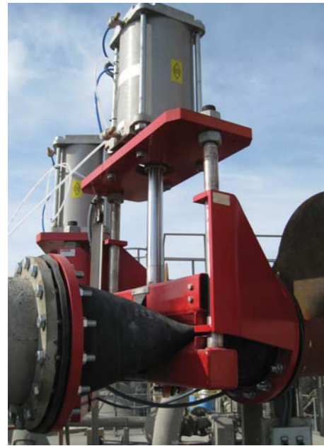
The pinch valve in pneumatic conveying.
